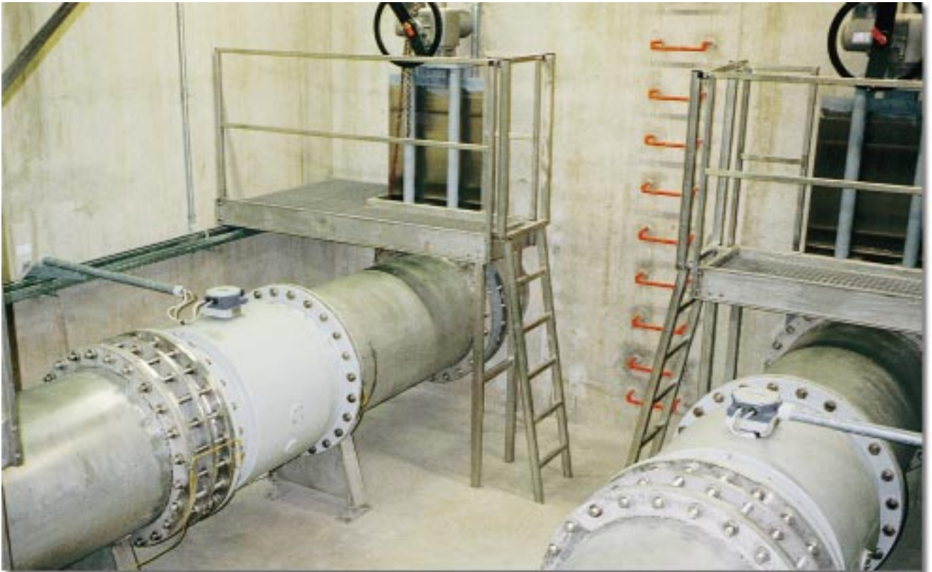
PARTI-MAG II, 2 meters DN 800 for dry weather flow metering and for outflow control of storage channels
